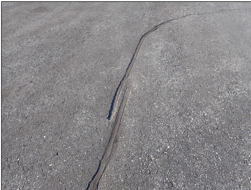
TW-05-13: L&T Cracking
