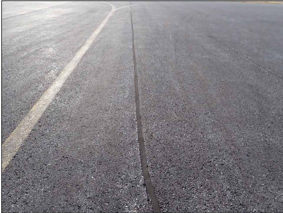
AP-11-17: L&T Cracking
