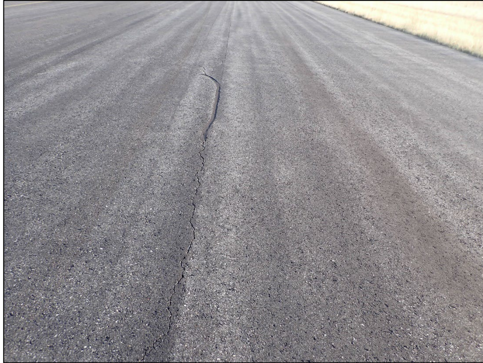
RW04-11-07: L&T Cracking
